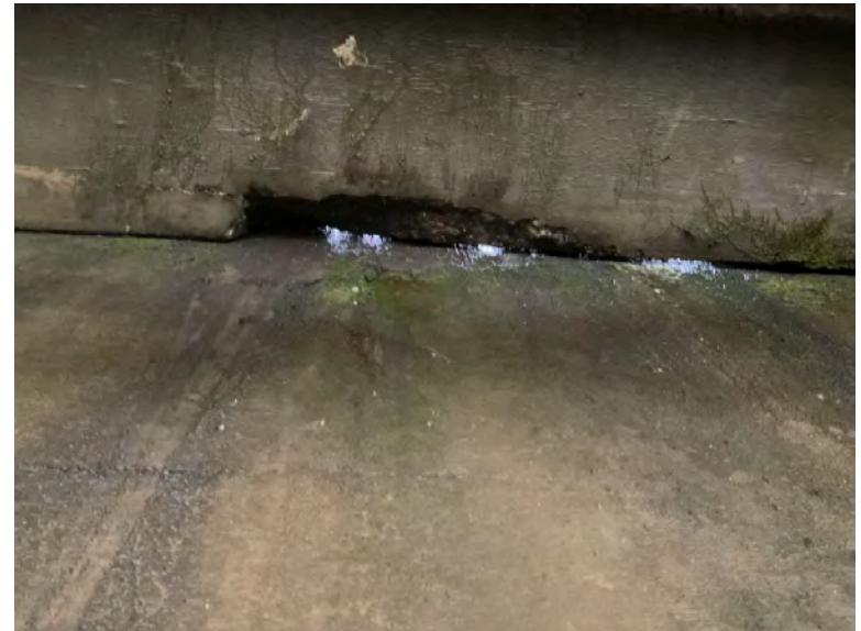
Damage to panel 1 right bank
