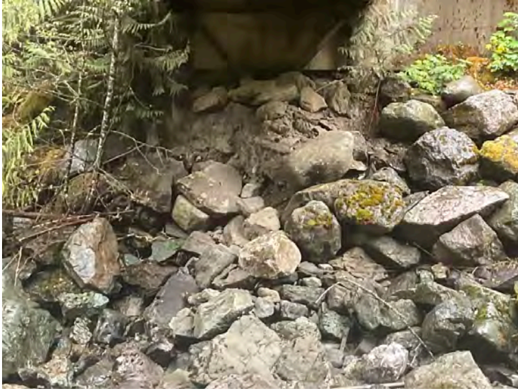
Right Bank Abutment riprap erosion
